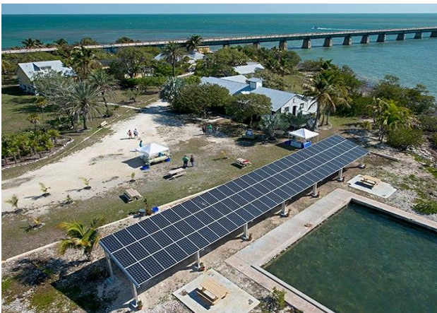
Pigeon Key Solar Panels - Monroe County, FL
